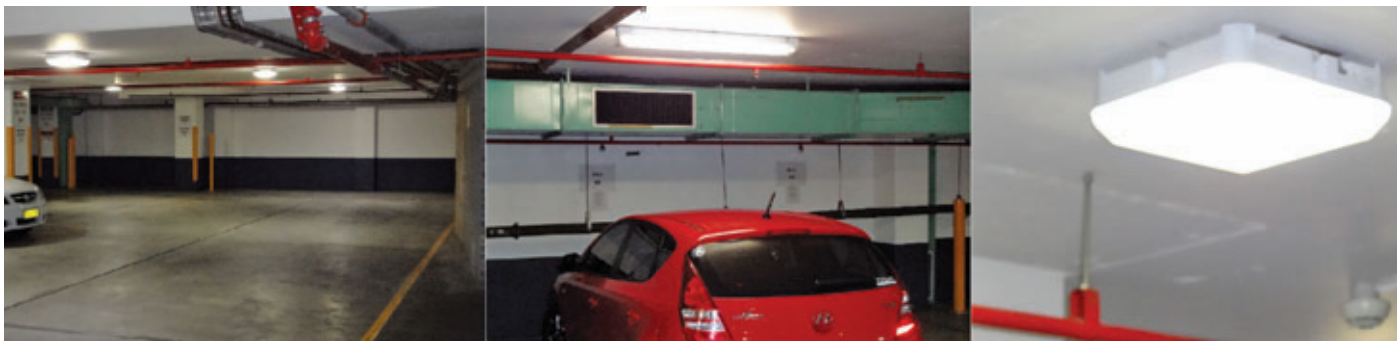
From left: Chamaeleon carpark occupancy mode; existing T8 carpark installation Chamaeleon lift lobby in occupancy mode.
